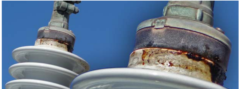
Picture 2: Leaking bushing turret
