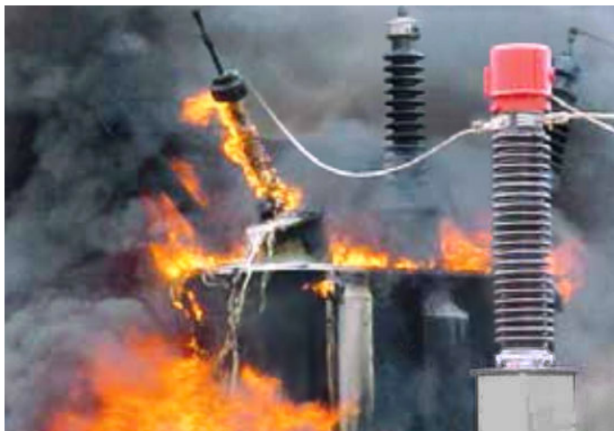
Picture 1: Fire as a result of a bushing fault: Oil / flames spread all over the tank [3].
